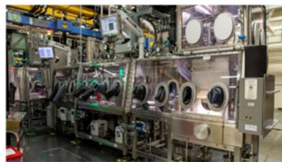
Electrorefining glovebox in the 9215 Complex.
